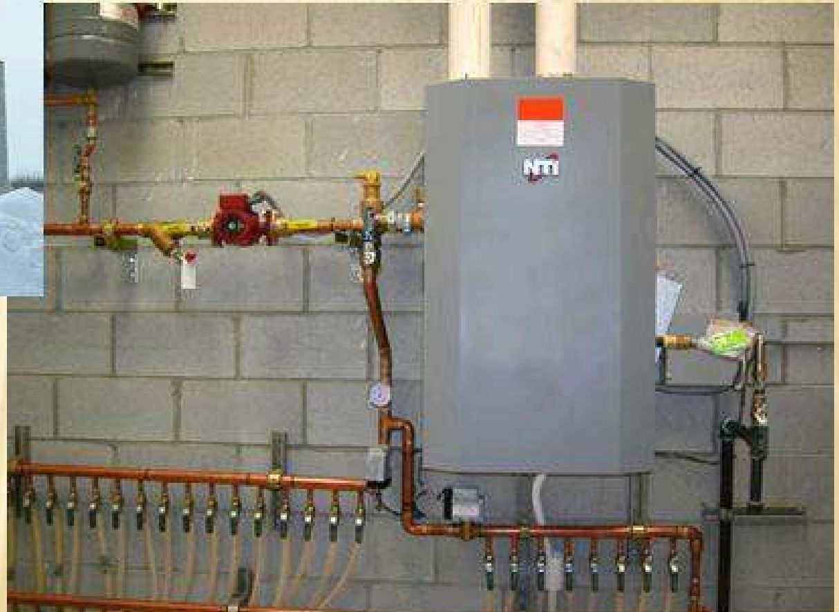
STARHEAT MECHANICAL ROOM
