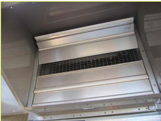
Relief dampers stuck open at Nvidia
