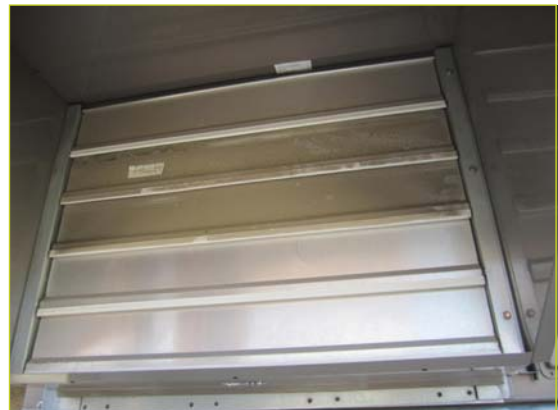
Dust on dampers gives clues to issues
