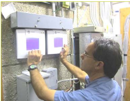
Programming rooftop unit heating/cooling controls
