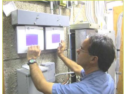
Programming rooftop unit heating/cooling controls
