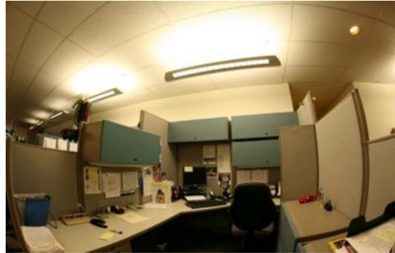
Cubicles lit with workstation-specific luminaires during the pilot study at the Philip Burton Federal Building.
